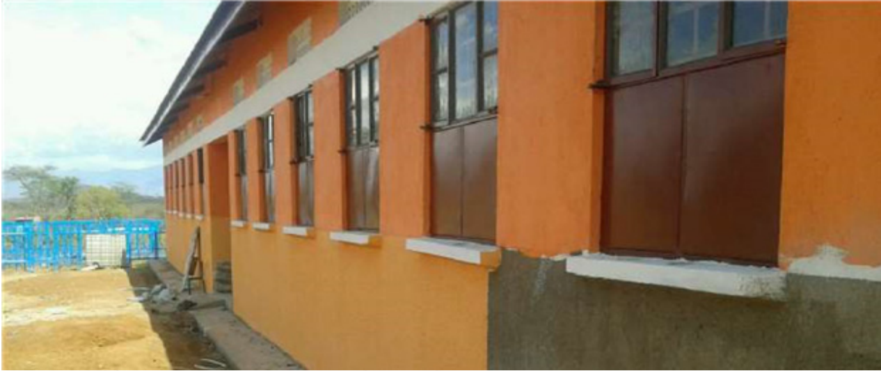
Fig 4: Completed dormitory at Kalikongel p/s – Napak District under NUSAF project office of the Prime Minister
